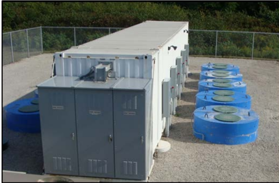
Figure 90. 1-MW Smart Energy Matrix Plant (Photo courtesy: Beacon Power)
