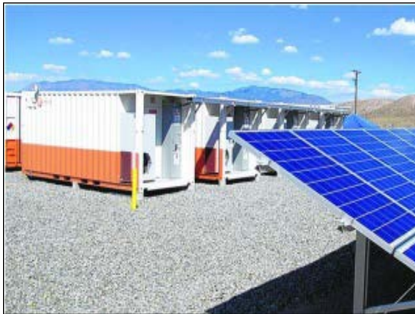
Figure 73. 500-kW/1-MWh Advanced Lead-acid Battery for Time-shifting and 900-kWh Advanced Carbon Valve-regulated Battery for Photovoltaic Smoothing This is a solar energy storage facility that is fully integrated into a utility's power grid. (Source: PNM Resources)
