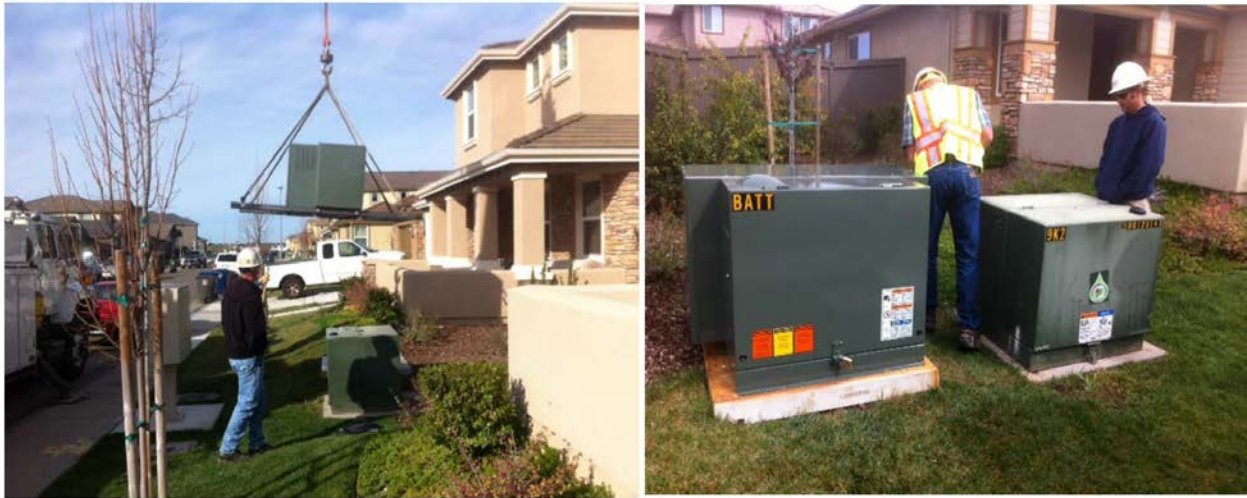
Figure 99. A 30-kW/34-kWh Distributed Energy Storage Unit (Being Installed and Inspected at the Sacramento Municipal Utility District's Anatolia SolarSmart Homes Development. Suppliers are SAFT, Grid Point, and Power Hub)
