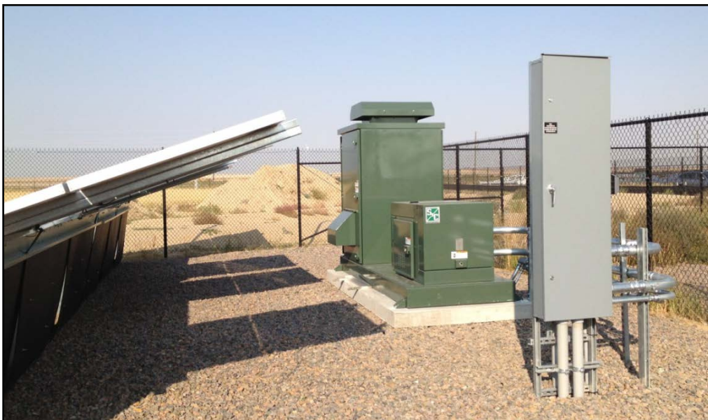
Figure 40. Containerized 25 kW/50 kWh FIAMM Battery Unit (large green housing) on Concrete Pad, Next to S&C PureWave CES (small green housing)
