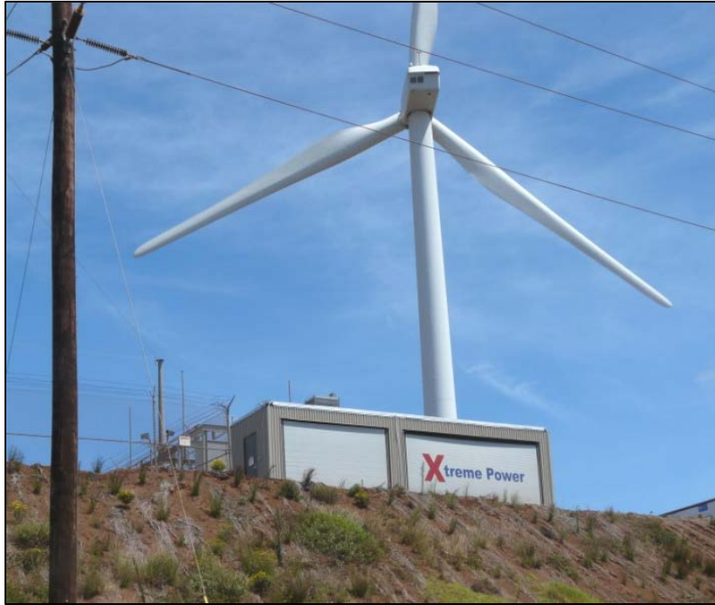
Figure 72. 1.5-MW/1-MWh Advanced Lead-acid Dry Cell Systems by Xtreme Power in a Maui Wind Farm (Source: Xtreme Power)
