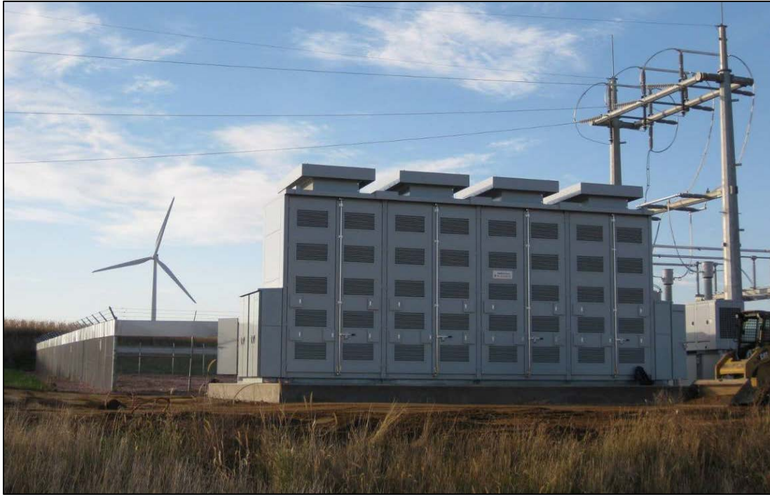
Figure 34. Xcel Battery Supplementing Wind Turbines, Lucerne, MN
