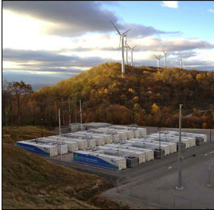
Figure 97. AES Storage LLC's Laurel Mountain Energy Storage (Supplies 32 MW of regulation in PJM using Li-ion batteries supplied by A123 Systems)
